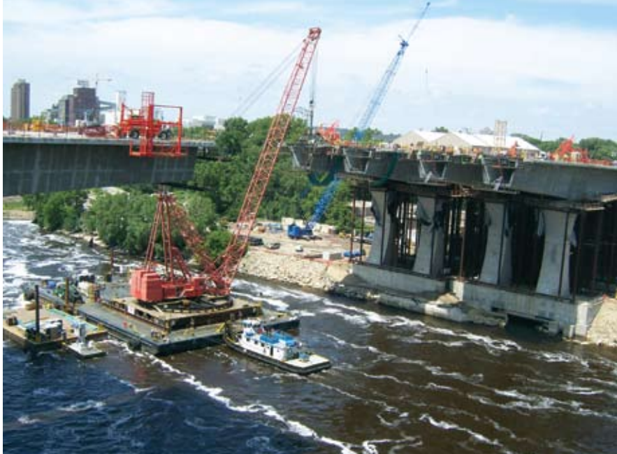
The segments were lifted into place using a 600-ton, barge-mounted crane. Photo: Mn/DOT.
